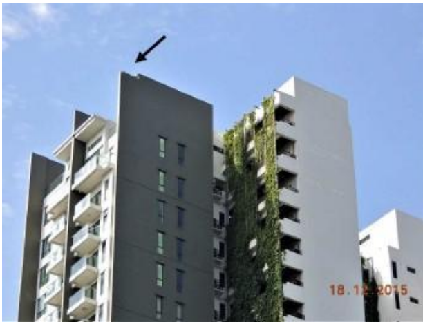
Figure 4 - Lightning damage on UNIV360 Place [11].
