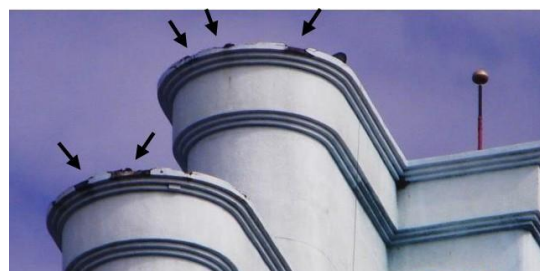
Figure 2 - Bypasses observed on a Malaysian building parapet a few meters apart from an ESE air termination [10].
