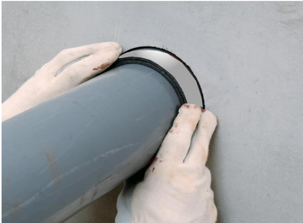
Figure 20: Pipe wrap fitted to pipe and being inserted in a concrete wall
