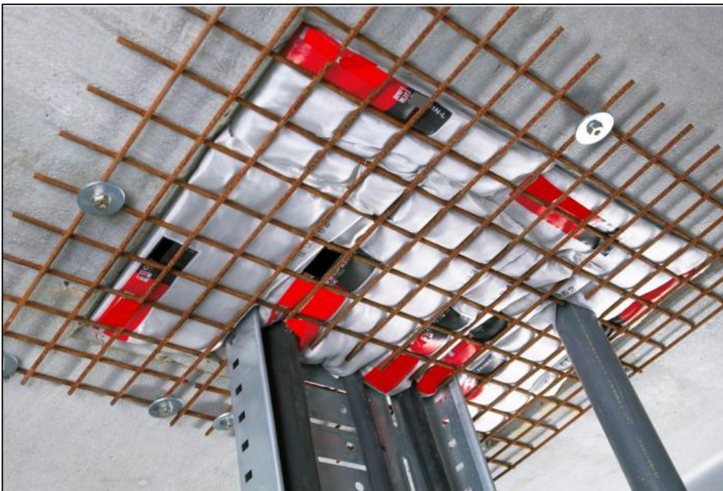
Figure 15: Pillows used to provide temporary fire-stopping of a vertical cable tray
