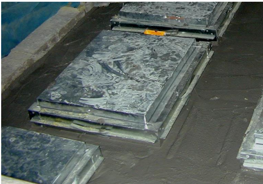
Figure 34: Fire damper fitted with expansion frame being sealed in floor opening with fire rated mortar. Note- damper in line with floor
